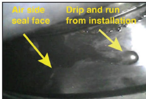
Figure 7: Excess Lube on Seam From Install
