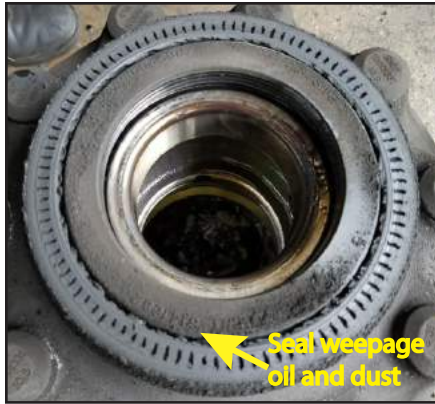
Figure 9: Acceptable Weeping Seal — Drum Brake
