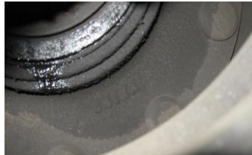
Figure 4: Leaking – Change Seal
